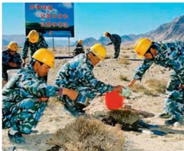
Grass restored. Grassland vegetation and its root soil layer were removed during construction then were replanted once the work was complete (12).
